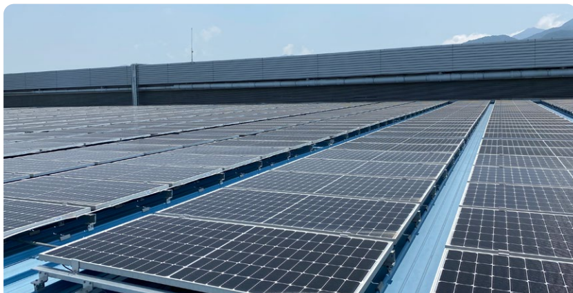
HAECO's PV system at HKIA consists of approximately 6,000 solar panels.
